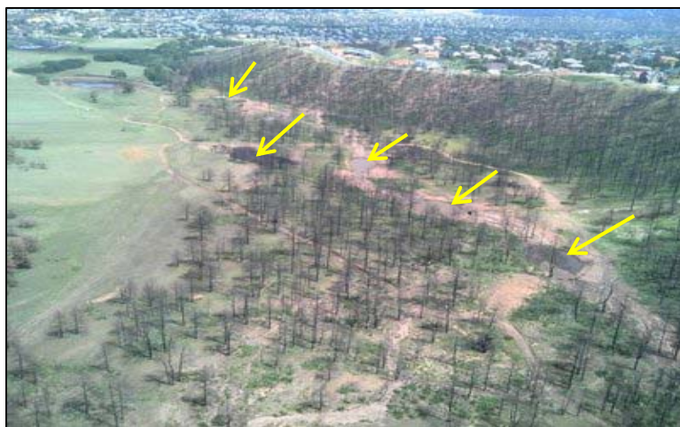
Figure 17 Post-construction of the five debris basins installed on North Douglas Creek on an alluvial fan.
