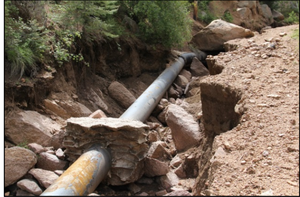
Figure 2 Damage to water transmission lines, North Monument Creek.
