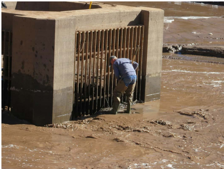
Figure 6 Manual clearing of intake tower trash racks to maintain open outlet works at Paonia Reservoir, November 2014
