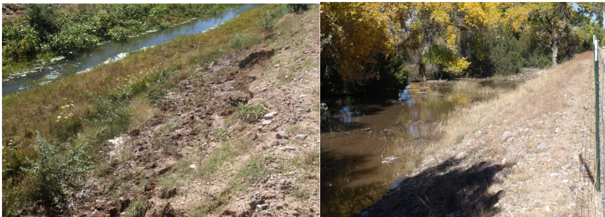
Figure 6 Seepage and pooling at the unconsolidated spoil levee. Left: Observed seepage on the landward side of the spoil levee. Right: Water pooled on the river side of the spoil levee. Photographs were taken on 9/26/2013 and 10/21/2013 respectively.
