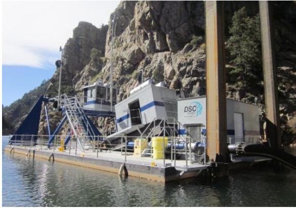
Figure 14 Hydraulic dredging of reservoir sediments for transport through a sediment slurry pipeline (Strontia Springs Reservoir, Colorado).
