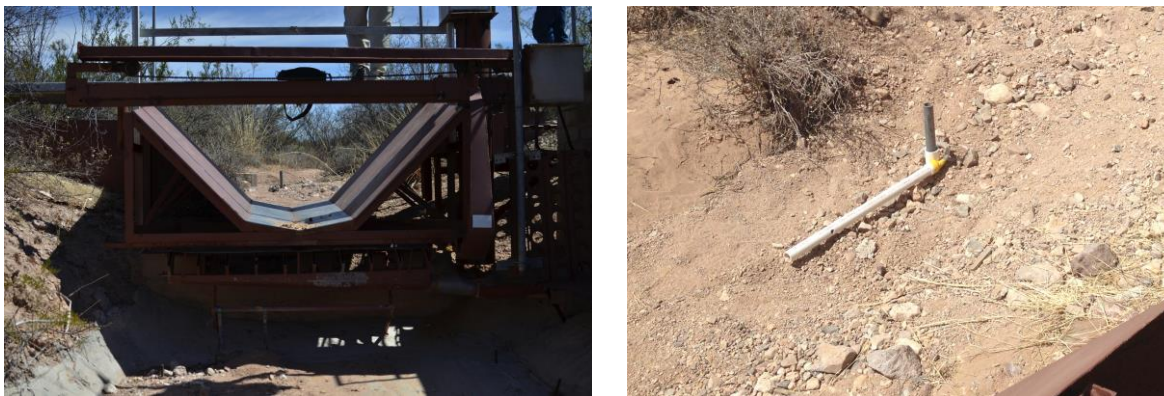
Figure 2 Left: The Santa Rita style flume at the outlet of Lucky Hills subwatershed. This view faces upstream from the outfall (where the pit sampler was later placed) toward the hydrophone mount (post seen in the upstream channel). Right: Photo of the PVC housing of the downstream hydrophone (mounting post visible in center of left photo).
