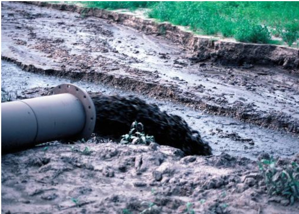
Figure 7. Sediment-laden water pumped as part of a dredging operation at Lake Panorama in central Iowa (Photo by Lynn Betts; Photo courtesy of USDA Natural Resources Conservation Service; Photo by USDA NRCS).
