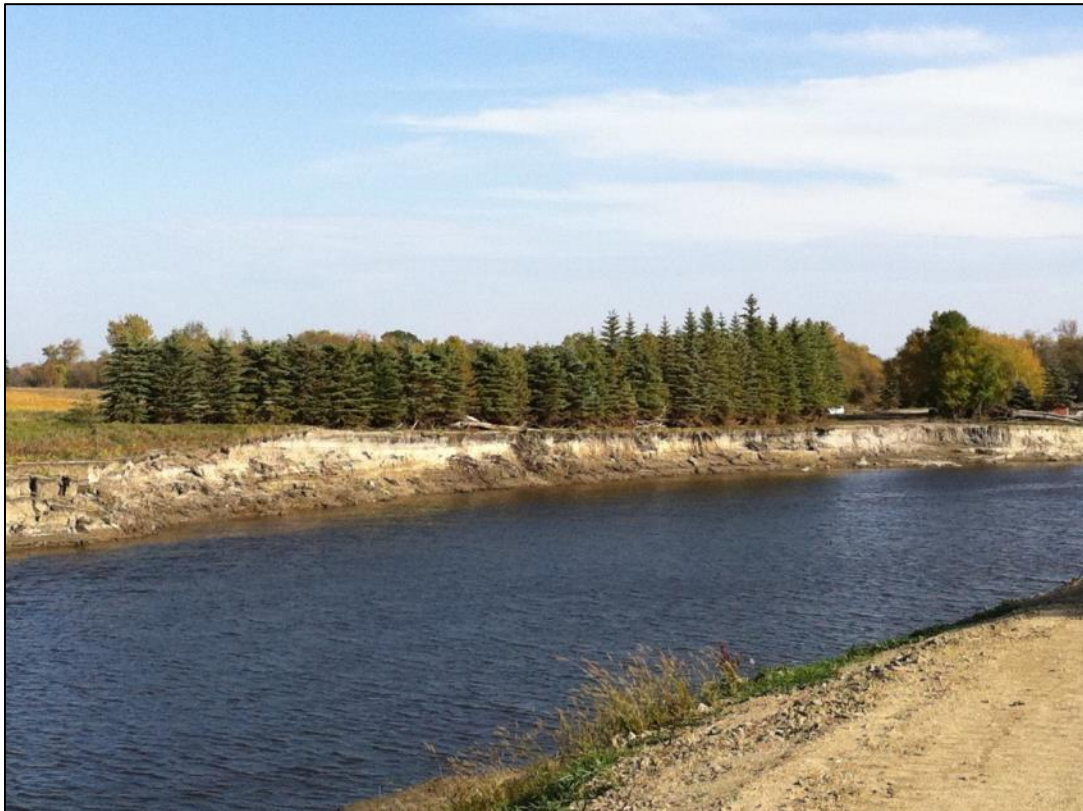
Figure 6 Significant erosion and channel migration after the 2011 flood opposite the existing levee at Velva.
