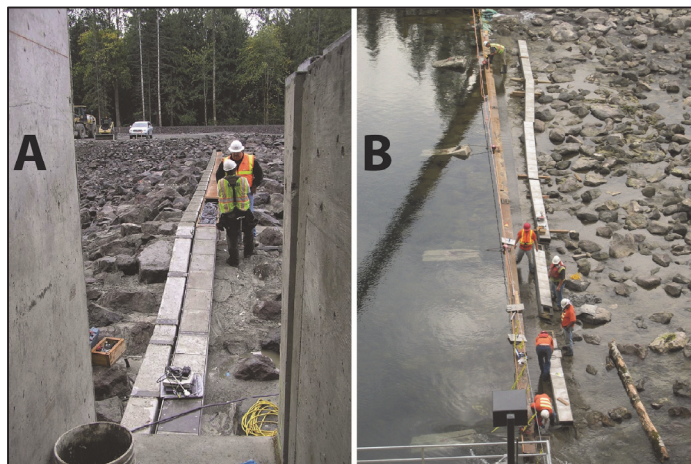
Figure 2 (A) 2008 installation of impact plates and sensors (#1 – #12) on river right, and wiring for the entire system. (B) 2009 installation of remaining impact plates (#13 – #72).
