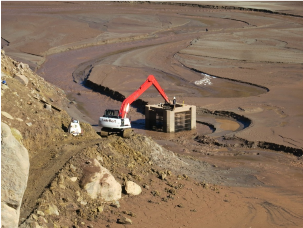
Figure 5 Long-reach excavator removing sediment and debris from intake tower at Paonia Reservoir, November 2014
