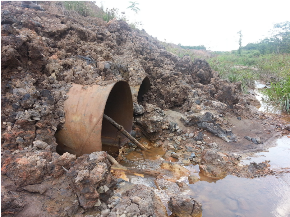
Figure 2 An eroded culvert crossing close to one of the mines
