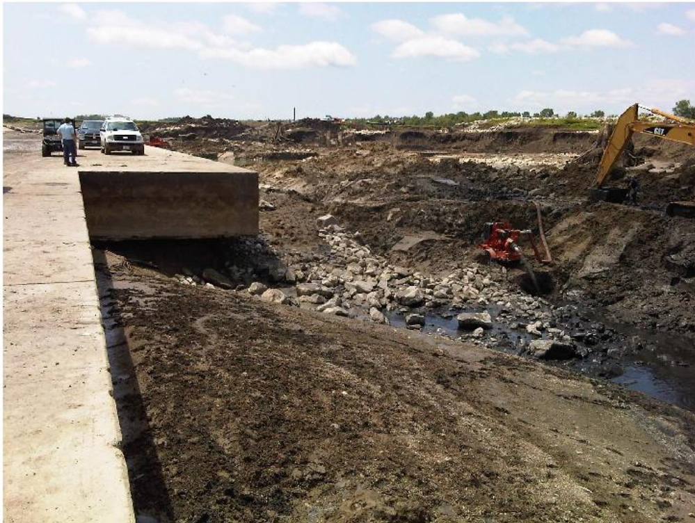
Figure 11 Scour Holes Downstream of the Plunge Pool's Extruded Corners
