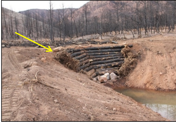
Figure 18 Newly constructed debris basin and crib wall on North Douglas Creek where the excavated material was used to fill the deep and wide gullies (note the arrow indicating the location of the rock and exposed root wad).
