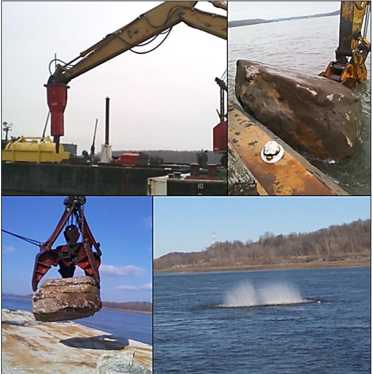
Figure 7: Rock was removed from the navigation channel using various means such as hydro-hammering excavating grappling and blasting
