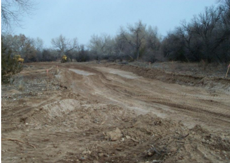
Figure 2 Constructing the side channel at RM 228.9 river maintenance priority site. Each path is the width of one tractor-scraper. Photo taken on January 30, 2008.
