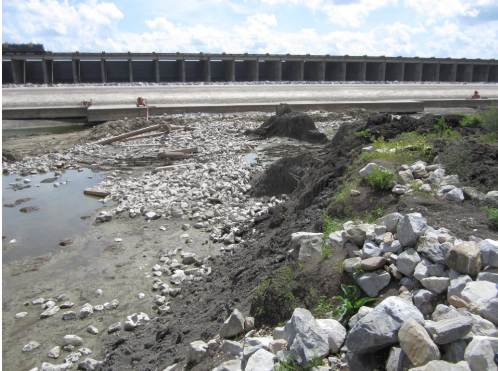
Figure 10 Scoured MCS Tailbay after 2011 Operation
