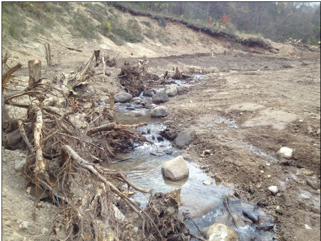
Figure 5 Upstream view of Bluff 1 in November, 2013, immediately after construction. Logs with root wads form one side of the channel and steps and pools were constructed in the channel.
