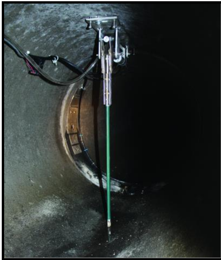
Figure 1 Image of the DISA in a closed conduit (storm sewer) with the sample arm extended in the vertical position. When at rest, the arm lies in the horizontal position near the pipe ceiling with the end of the intake pointing in the direction of flow. The sample arm (identified as green in this photo) can be sized to fit various conduit diameters. Photo by USGS.
