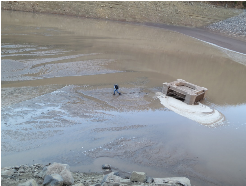
Figure 2 Sediment deposition at Paonia Reservoir outlet works intake tower, October 2014
