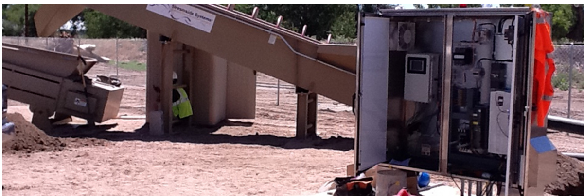
Figure 5 Electronic control panel and Archimedes screw separator.
