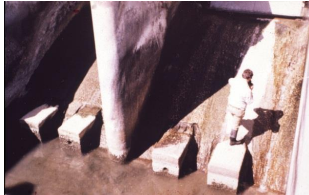
Figure 5 Sand has abraded the spillway at the Milburn Diversion Dam near Sargent, Nebraska.
